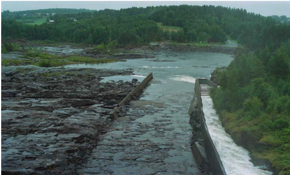
Figure 8. Spillway channel is comprised of rough, unfinished bedrock. The first energy-dissipating basin is downstream by the fish ladder entrance.
